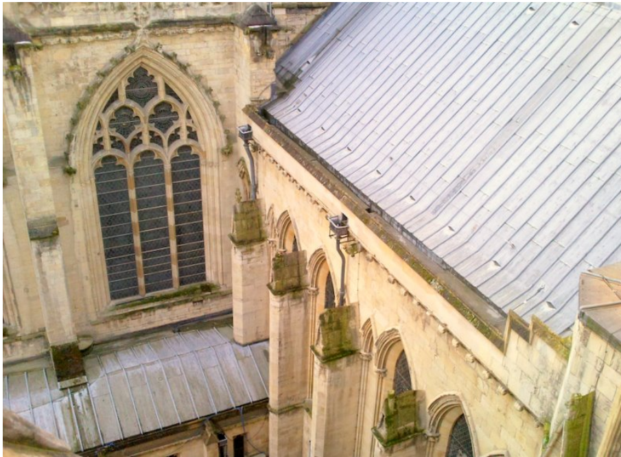
North Choir Aisle outbuilding in the angle between the North and East transept (credit:author)
