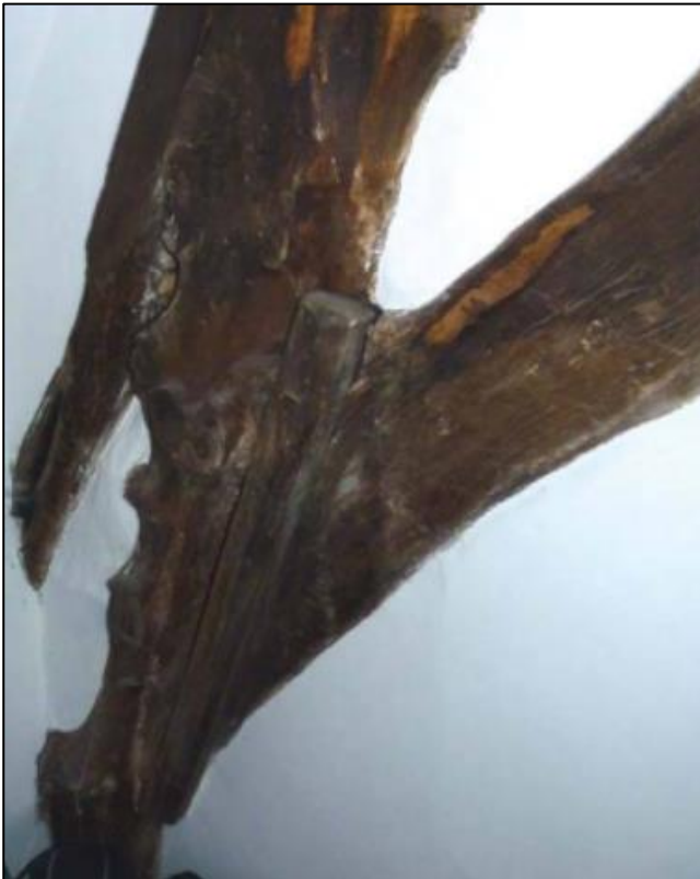
Figure 5: 1-2 Ufton north side of one of the trusses, still exposed to this day. This is a clear expression in the earlier open phase of the house, which in many other houses was later purposefully hidden (Alcock & Miles 2012, 21).
